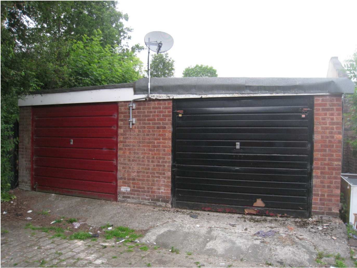
Satellite dish on roof of garage
